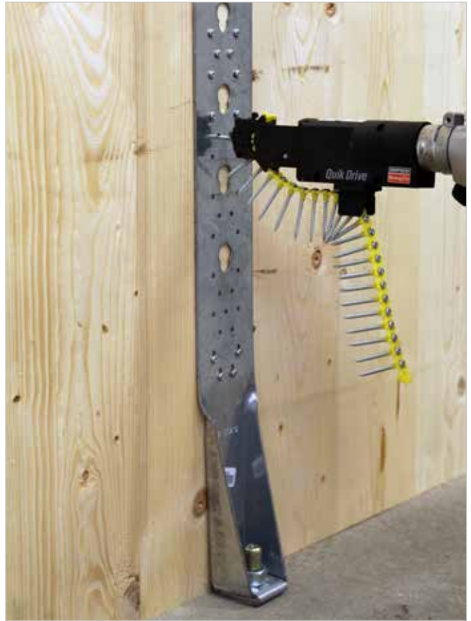
Quik Drive collated CSA screws fastening HTT31 holdown in CLT wall to concrete slab installation.
